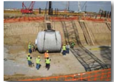
Crews install the first circulating water pipe at the Prairie State Energy Campus.
