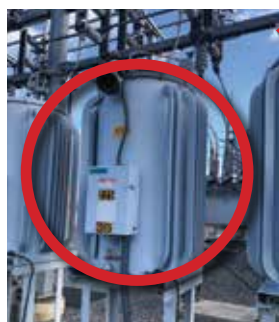
This regulator was found to be arcing internally. A report is submitted online with the location of the deteriorated equipment and a photograph.
